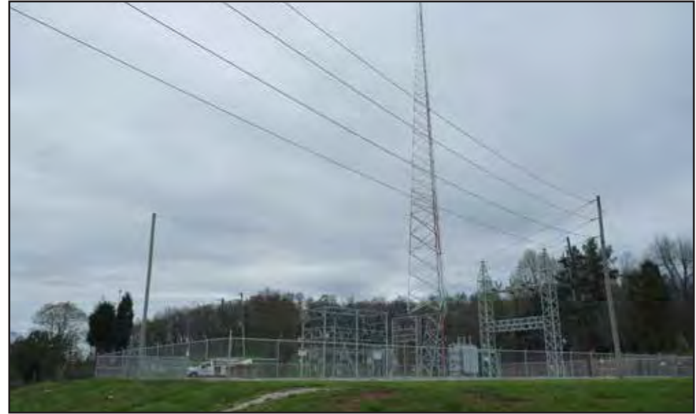
Photo 30: Existing utility; electrical substation; facing northeast.
